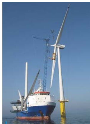
Offshore wind turbines Eoliennes offshore
